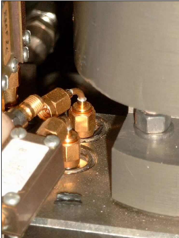
Fig. 2: BPM during the disconnection process.
