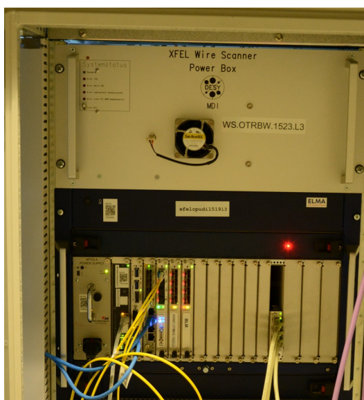
MTCA system (bottom) and Power box (top), latter is a 5HU 19inch box installed in an EXFEL rack
